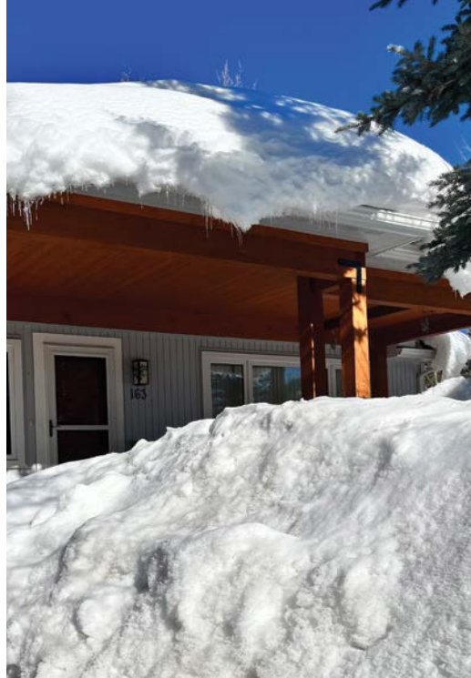
A heavy buildup of snow and ice on this pitched metal roof highlights the risk of sudden rooftop avalanches, emphasizing the importance of installing a properly engineered snow retention system.
