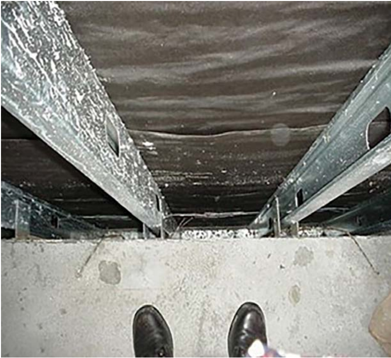
Gap between curtain wall and edge of slab.
