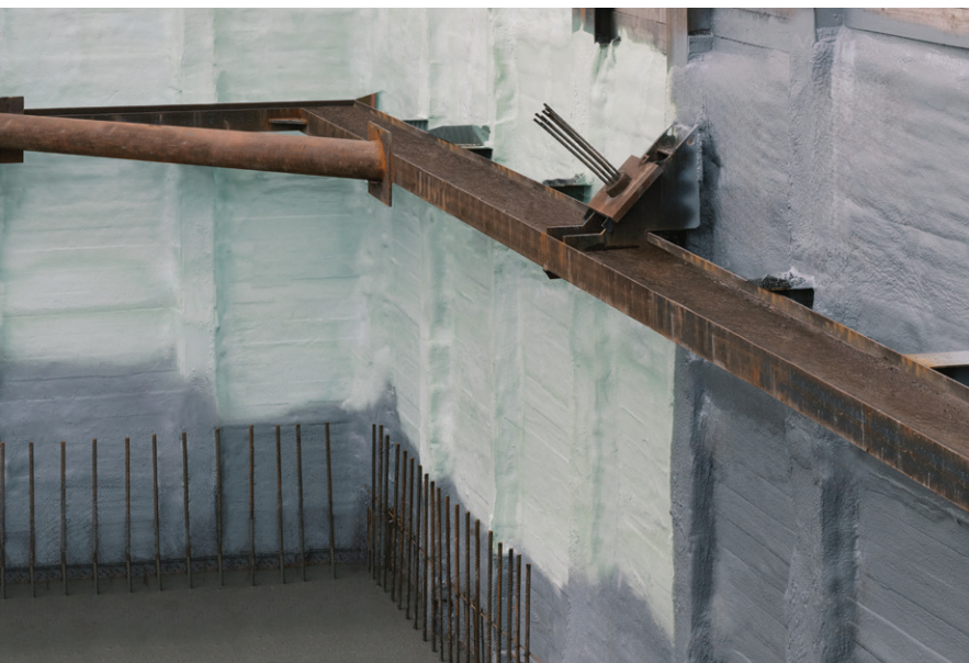
The foundation waterproofing project during polyurea coating application over closed-cell spray foam.
