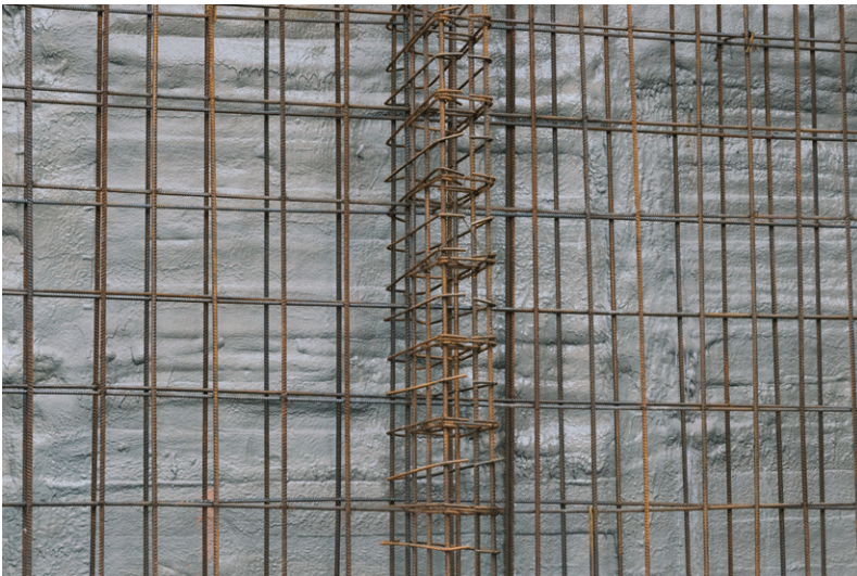
Grid of steel rebar over the waterproof coating and closed-cell spray foam insulation to enhance durability and resistance to environmental factors.
